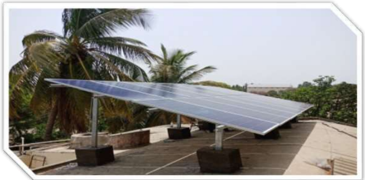
5KW Solar project at Principal bungalow
