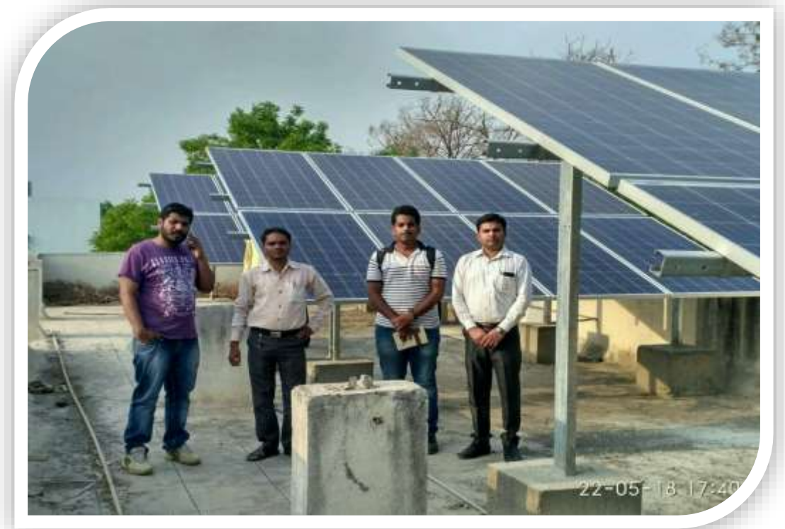
10 KW project Jain Solar at Girls Hostel
